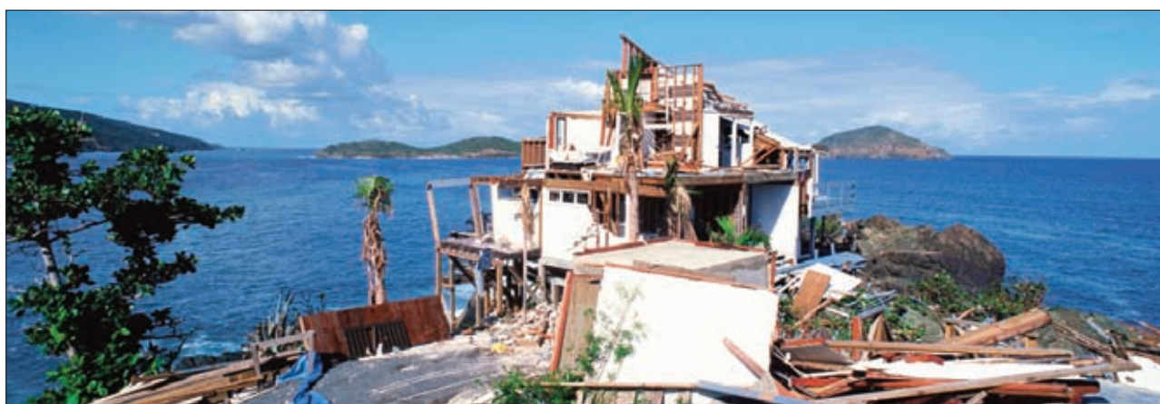
Destruction after hurricane
